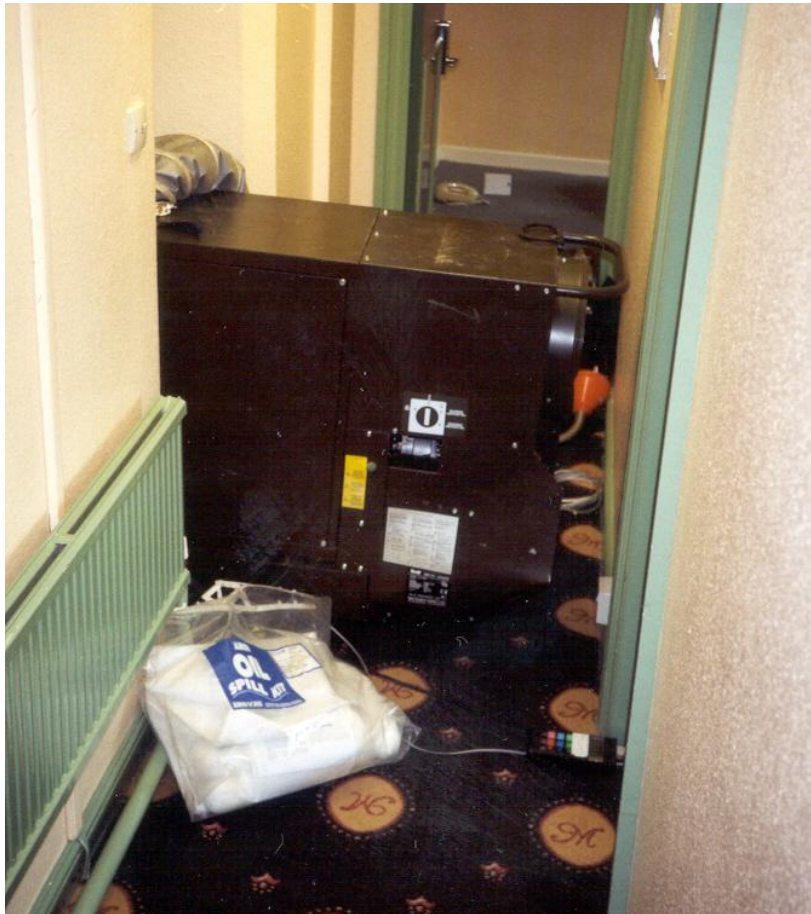
50kW heating unit powered by 230v single phase supply and diesel, fumes from which vented via 30m of exhaust ducting.
